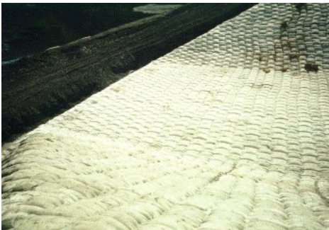
Entrance point of the spillway. ABM mat is buried in a 10 feet deep trench at this location.
