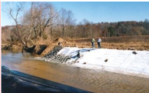
ABM panels being inflated on the inside embankment. Note the geotextile filter fabric on the slopes of the outer embankment in the foreground.
