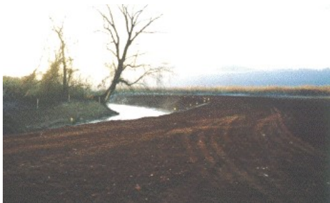
After grading was completed the creek was effectively "moved" to re bury the exposed pipeline. Also note that the electrical tower is now far away enough from the outer embankment to be out of the photograph.
