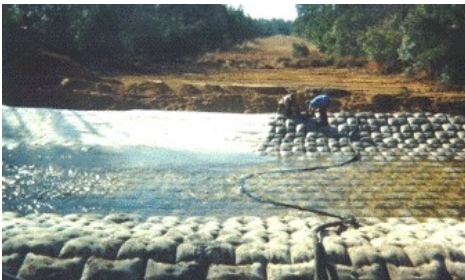
ARMORFORM ABM being installed over a fiber optic cable crossing in a shallow creek.
