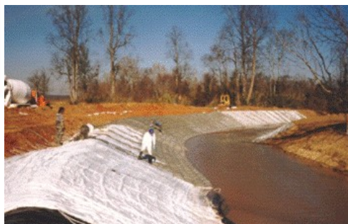
As the inflation of the ARMORFORM mats continues into the second day a dozier can be seen in the background filling in the anchor trench of the mats installed the previous day. Note the change in the color of the concrete. The freshly pumped concrete in the foreground is dark gray, while the concrete that was installed the previous day has turned to a whitish color.
