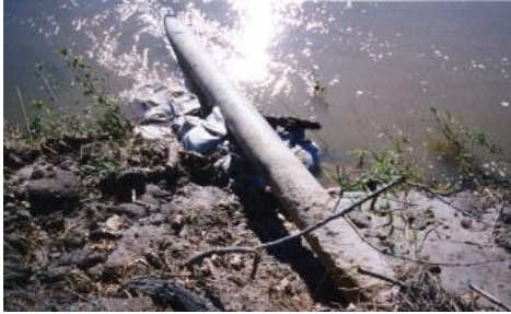
Exposed 16" diameter pipeline caused by the natural relocation of Raccoon Creek.
